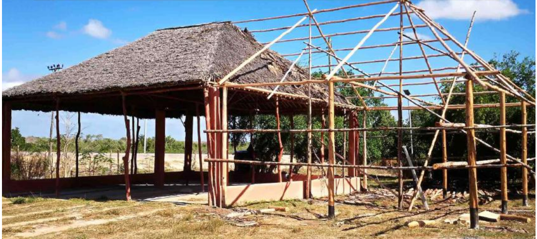
The TRLF Emmaus centre employs a mix of traditional and modern building technologies for sustainability
